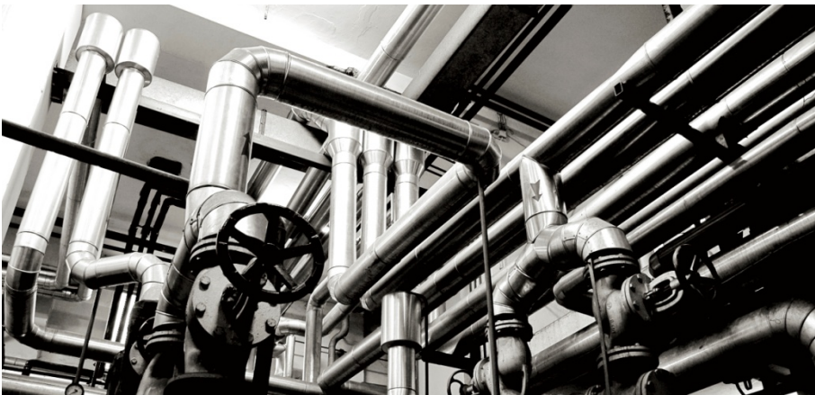
Pipeline Monitoring (Leakage Detection)
